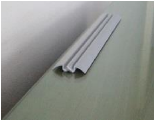
Aluminum threshold for sliding doors, not weather proof.
